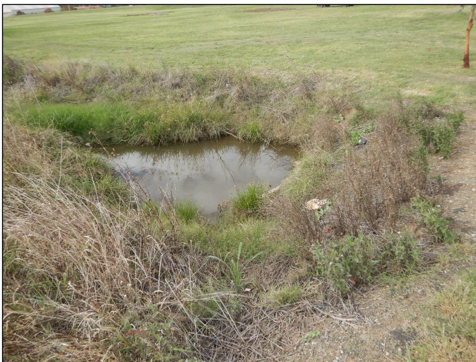
Figure 9: View of ponded water within southern part of swale drain
